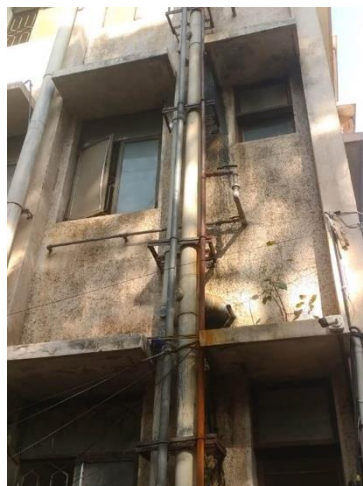
Figure 4-11: Waste water pipeline
