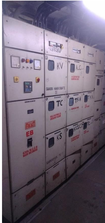
Figure 5-2: Main distribution panel
