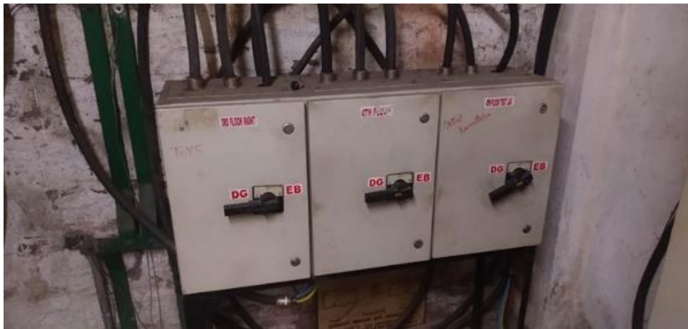
Figure 5-5: DG changeover switch
