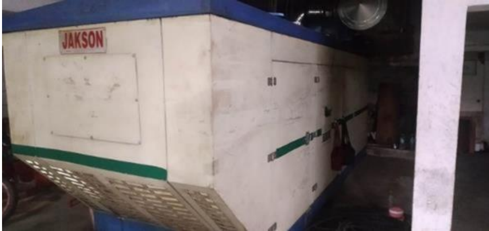
Figure 5-4: Diesel Generator (DG) Set
