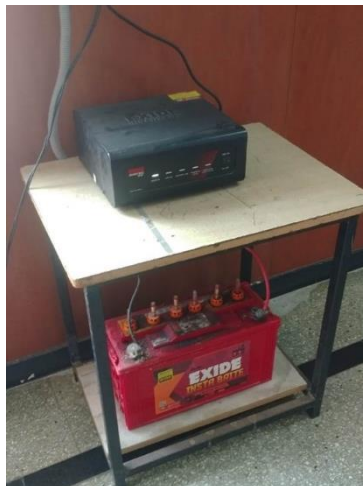
Figure 5-6: UPS in the college
