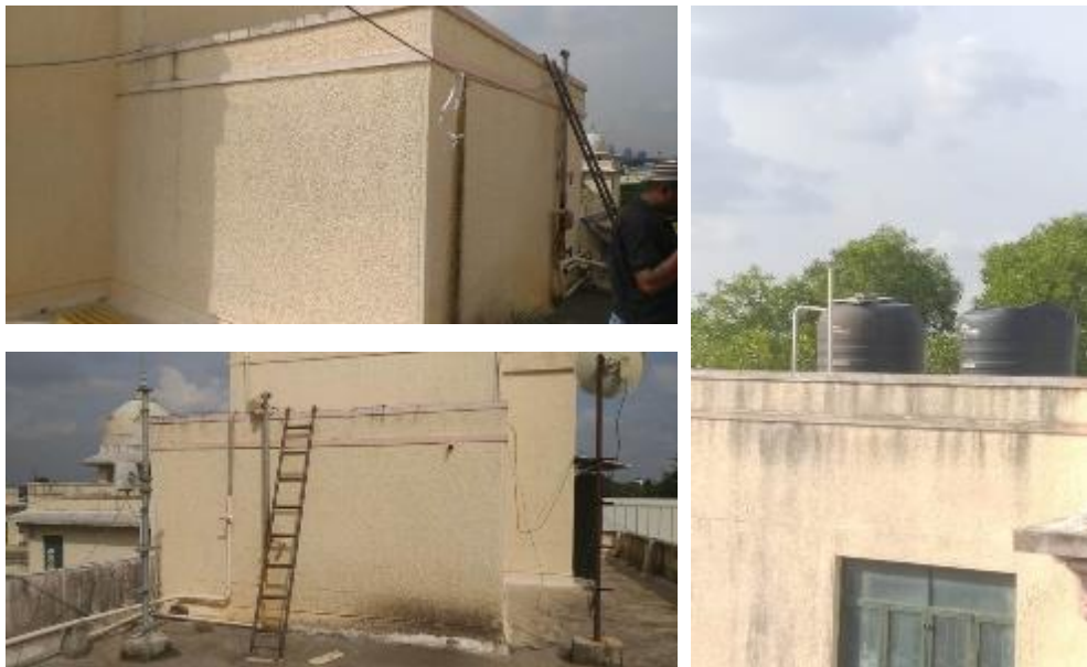
Figure 4-4: RCC and PVC overhead tanks
