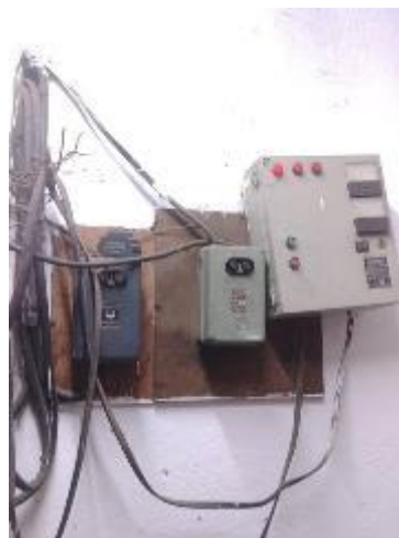
Figure 4-2: Borewell motor starter panel
