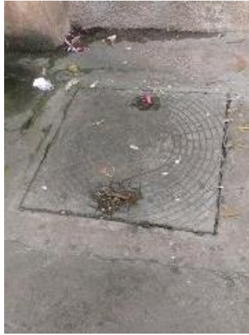
Figure 4-12: Waste water chamber
