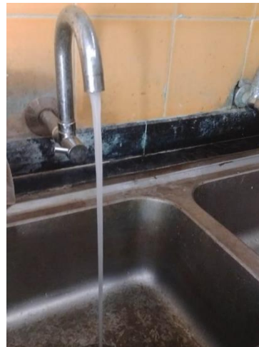
Figure 4-14: Aerator taps used in canteen
