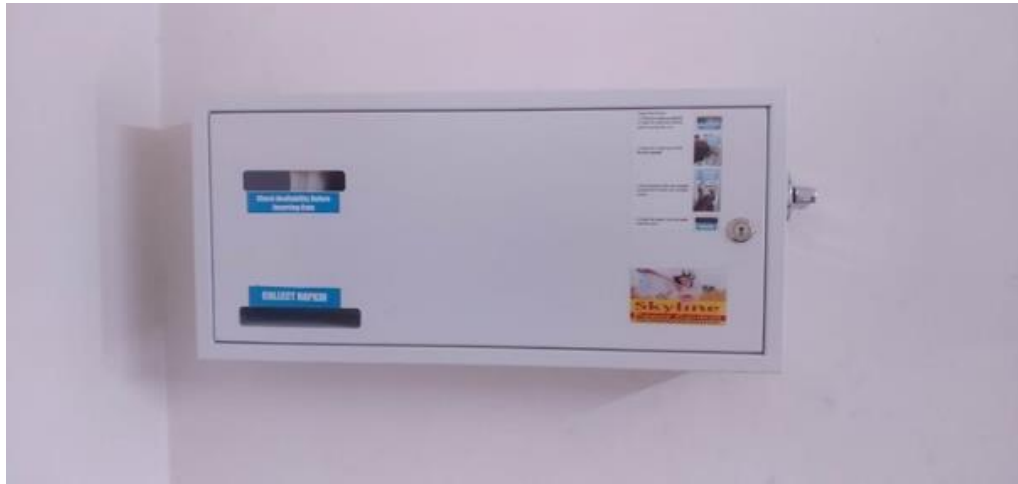
Figure 6-1:Sanitary hygiene napkin dispenser at 4 th Floor Girls rest room
