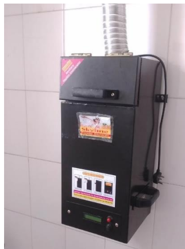
Figure 6-2:Napkin Incinerator at 4 th floor girl's rest room
