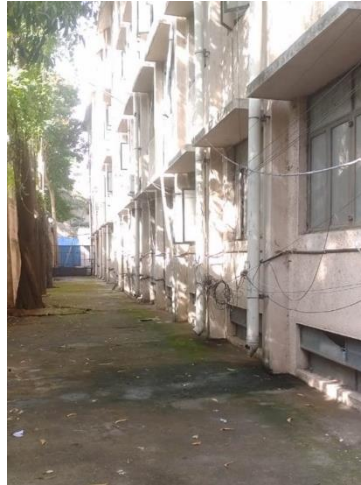
Figure 4-8: Rain water outlet pipelines
