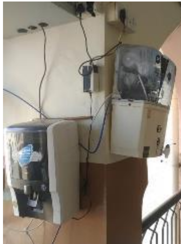
Figure 4-7: RO purifiers installed in the college
