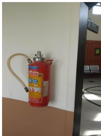
Figure 3-1: Fire Extinguisher at college premises
