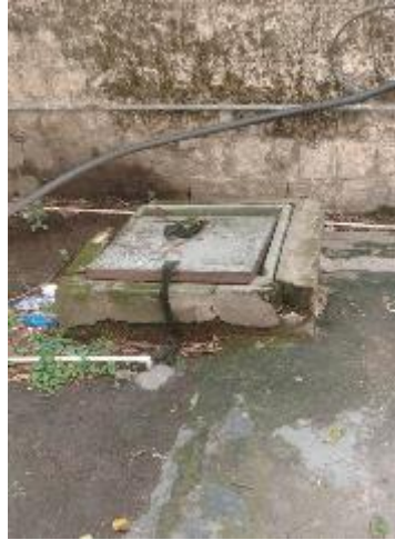
Figure 4-3: Raw water sump
